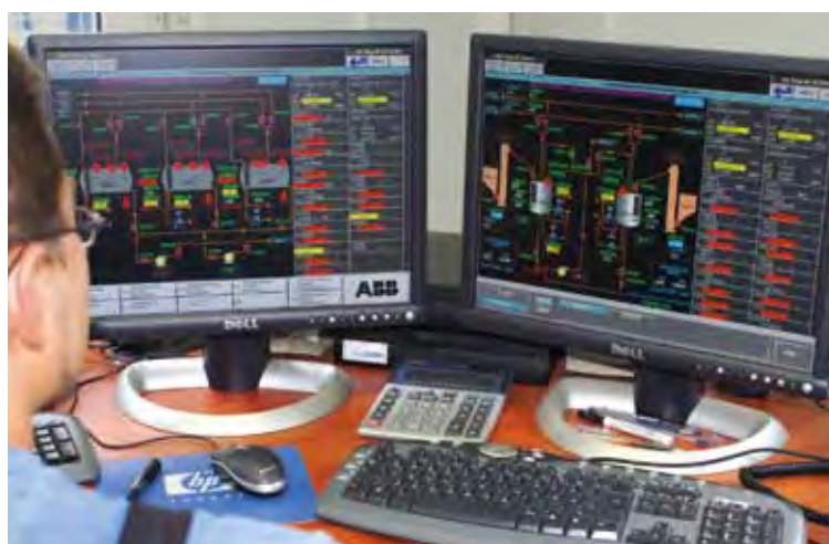
Figure 1.4. DCS system for the Płock site ORBITON modified bitumen production (photo by ORLEN Asphalt)
